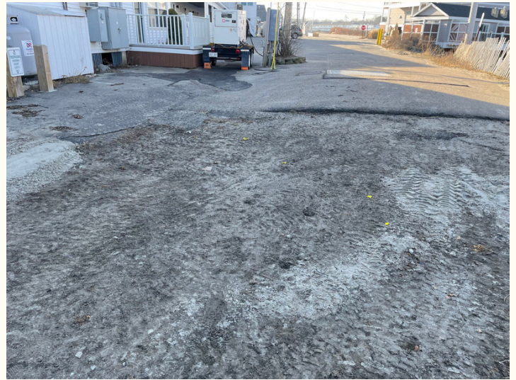
Condition of the street looking from the dunes/estuary toward the beach parking lot
